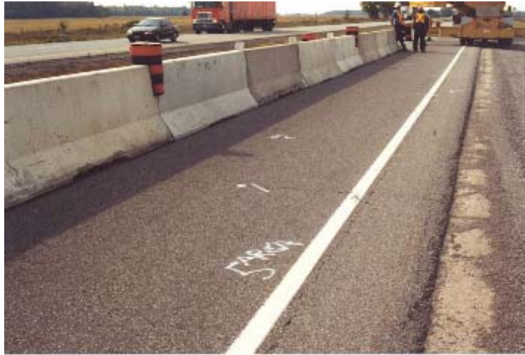
Figure 1. Typical pavement condition in eastern PMS sections
