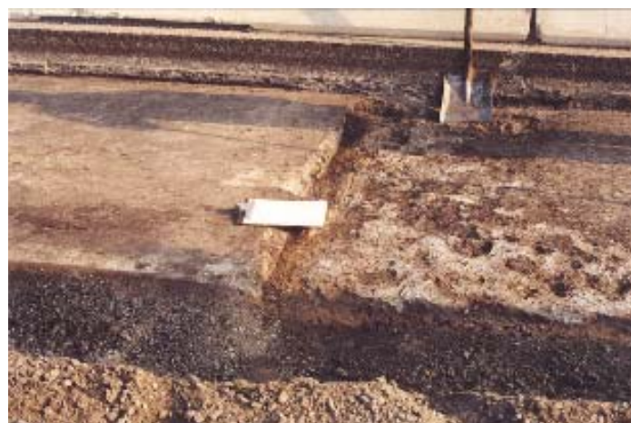
Figure 5. Severe concrete road base faulting.
