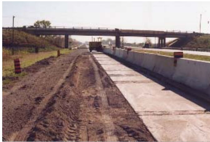
Figure 3. Typical concrete road base condition in western PMS sections (near Windsor). Note evidence of previous crack repair.
