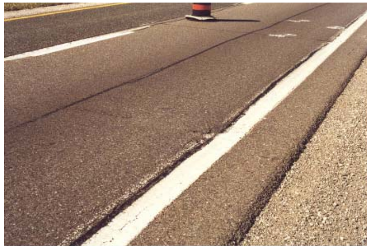
Figure 2. Typical pavement condition in western PMS section
